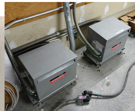
Transformers stepping down from 600~480V.
