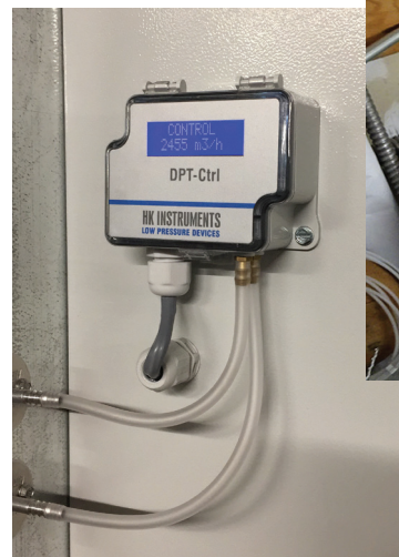
Standard Differential Pressure Controller with Pneumatic Signals
