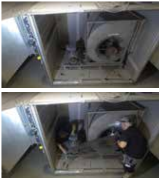
A. Before- AHU with Inefficient Belt Driven Fan
